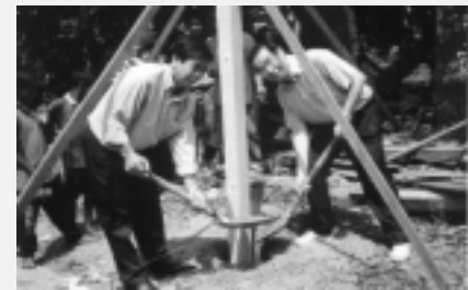
UPON THIS PILLAR SHALL THE CHURCH STAND: Pr Richard (left) and Pr Dr Chew securing the foundation pillar at the groundbreaking ceremony to mark the start of work on the new building.
